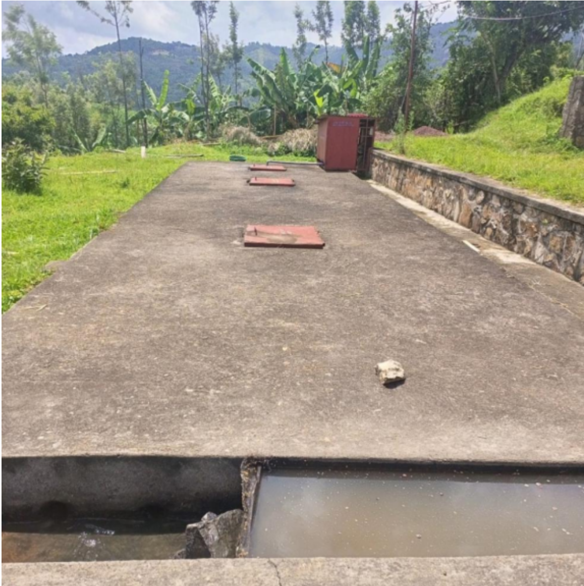
Figure 6: Bio-digester system of Kopakama Cooperative in Rwanda
